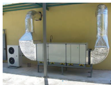
D-Air conditioning unit
